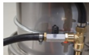
Compressed air distribution with compressed air diaphragm pump
